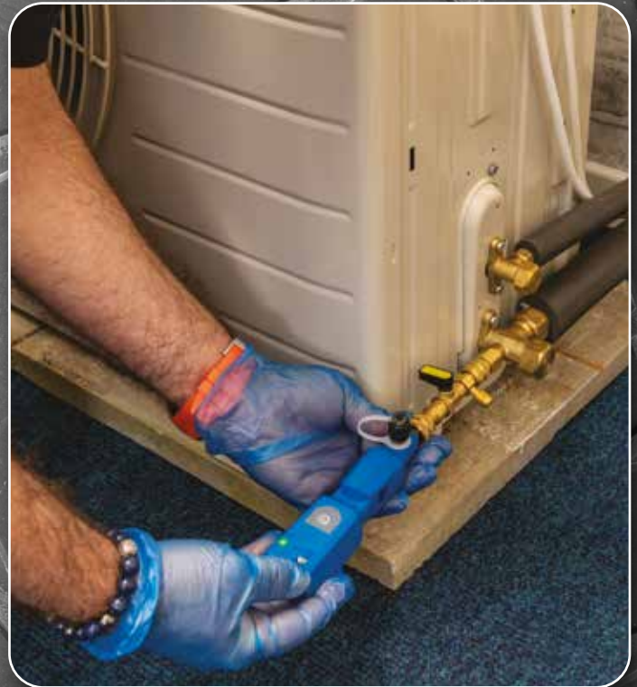
Wireless temperature & pressure measurements
