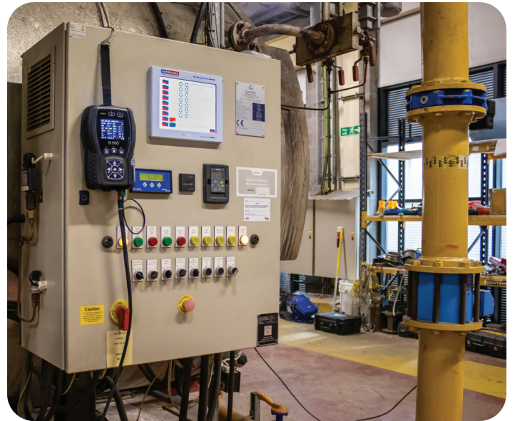
Industrial Boiler Analysis
